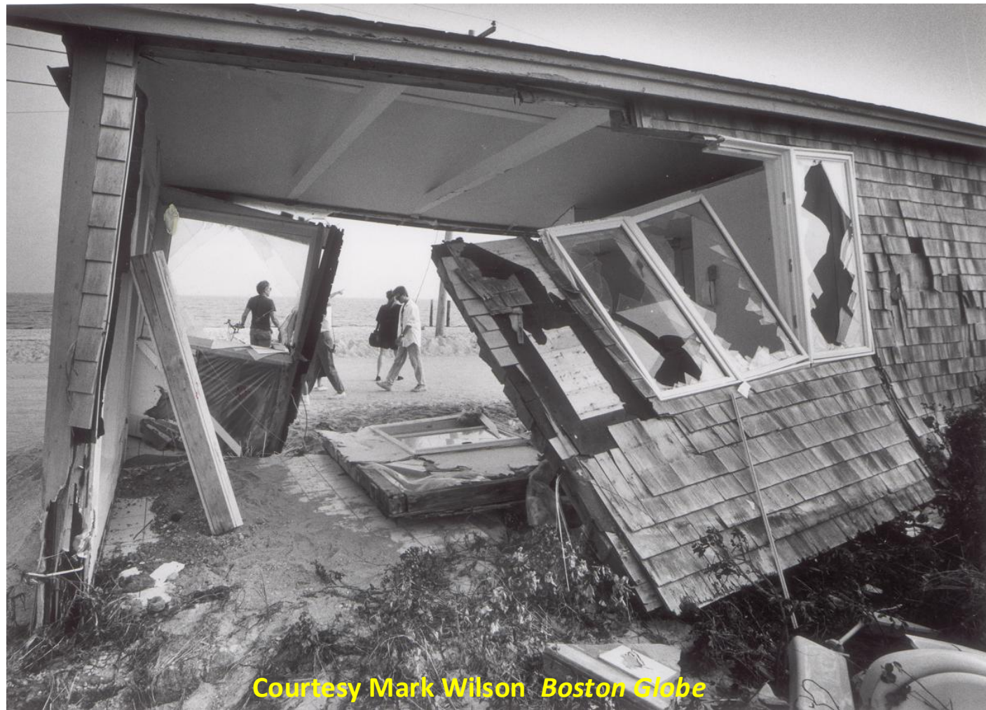
Cottage moved off foundation in Falmouth across Surf Street
