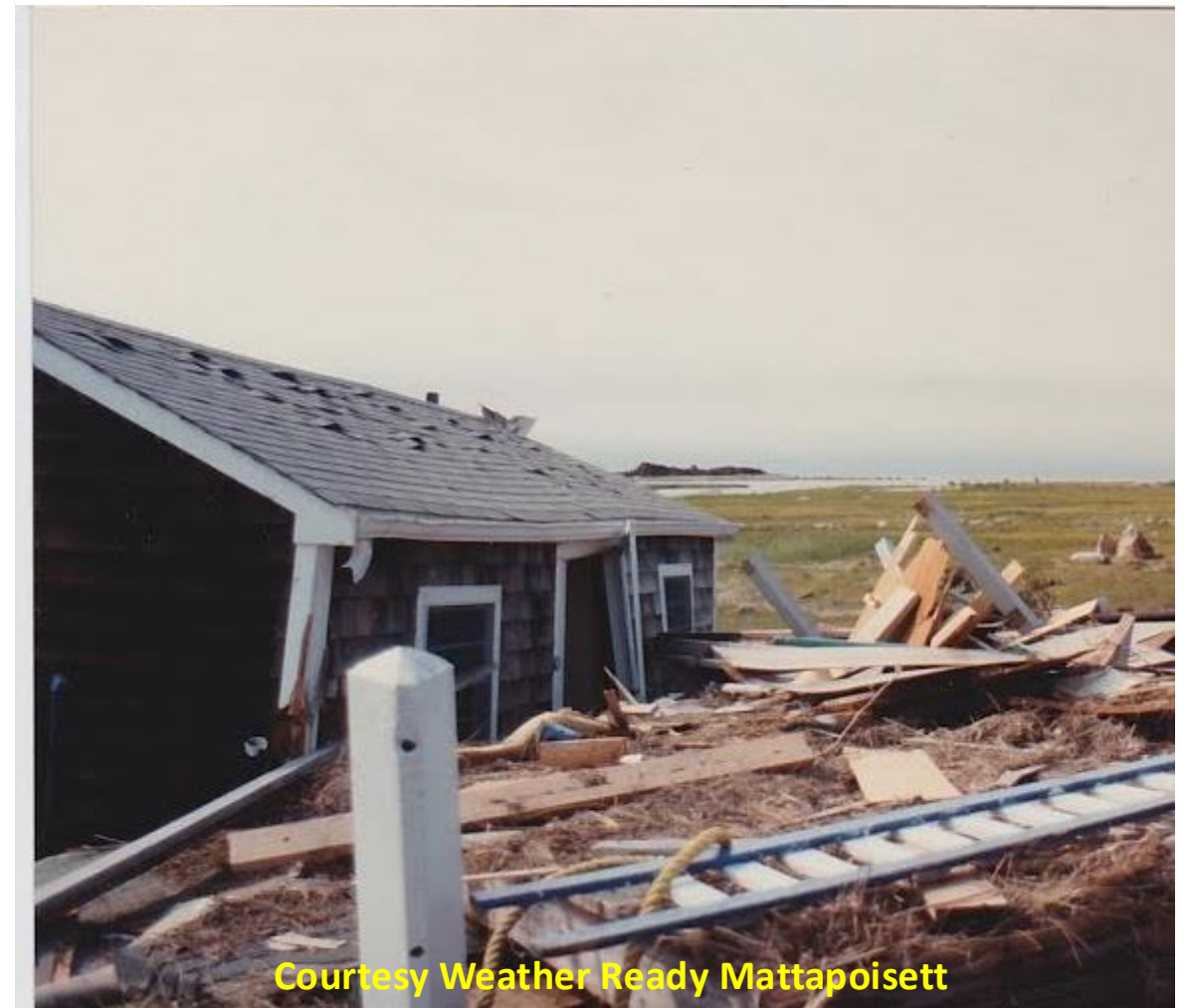
Mattapoissett, MA after Hurricane Bob
